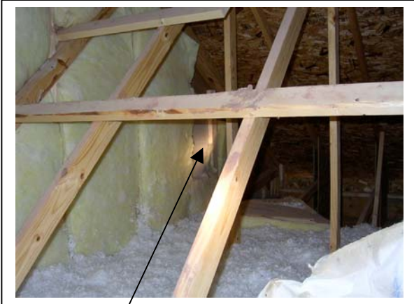
Fallen insulation at loft stairs area.
