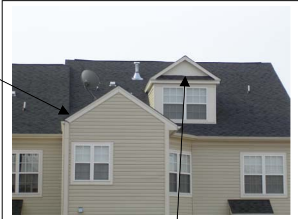
Potential vulnerable areas at rear roof.
