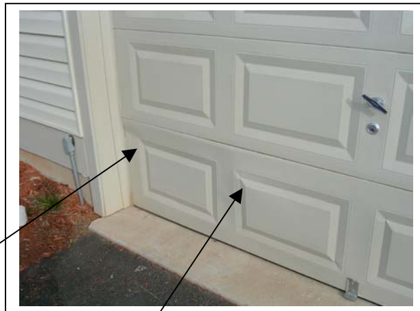
Damage at garage door.
