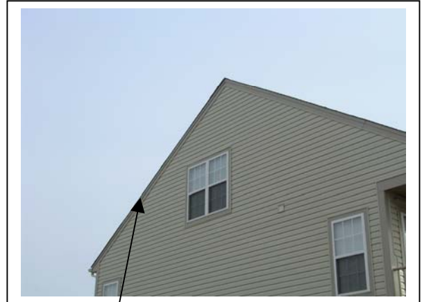
Roof trim needs caulking.
