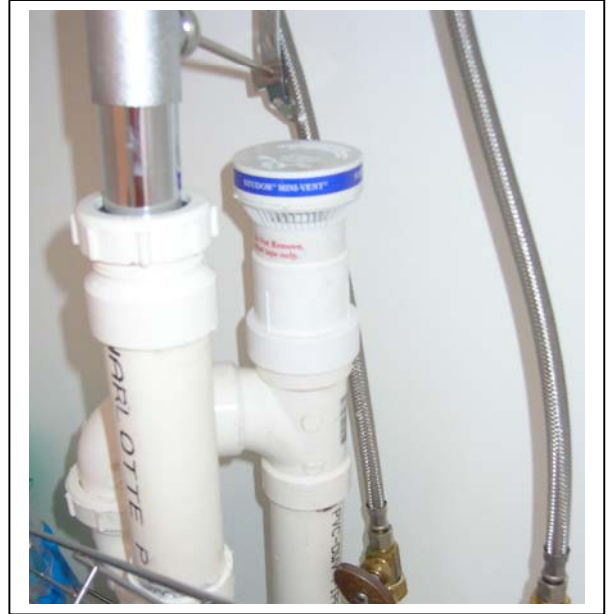
Mechanical vent at kitchen sink.
