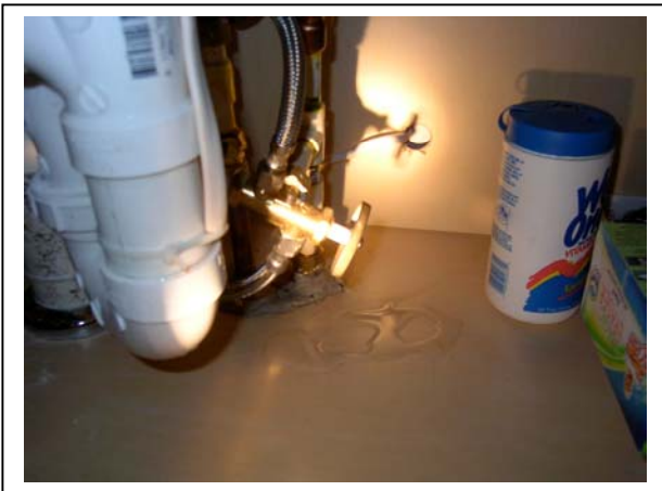
Leak under kitchen sink.
